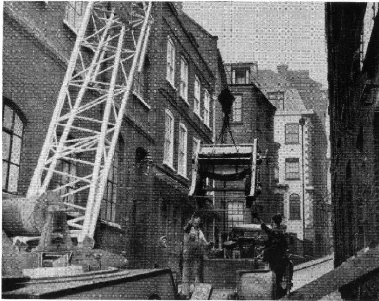
Not a mangle, but a 30 cwt. press being lowered by the crane.
