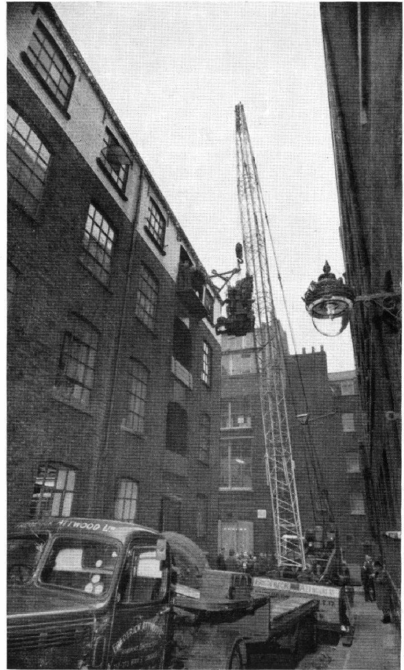
Another machine is hauled out from the 4th floor by the enormous crane.
