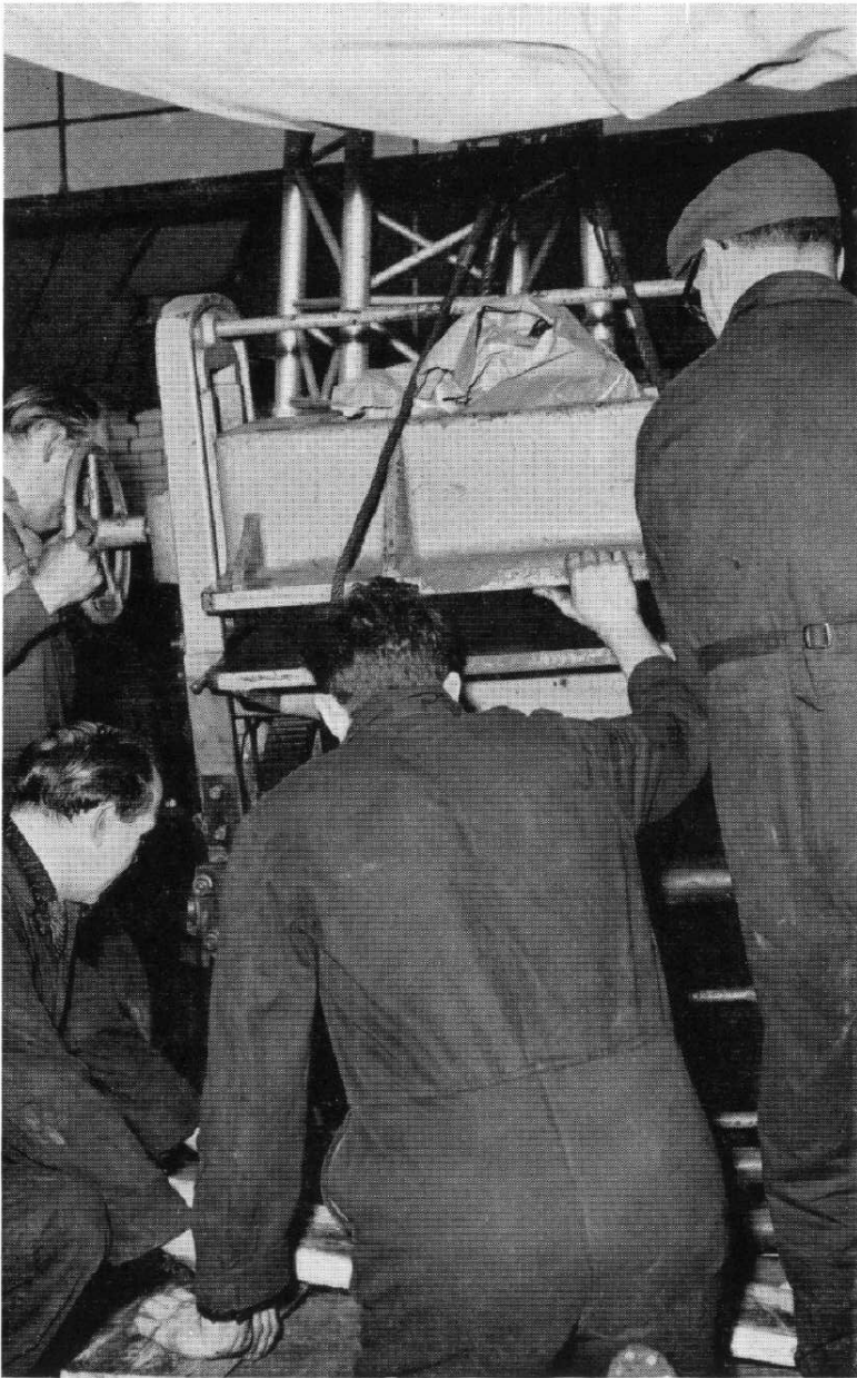
Out through a hole cut in the side of the roof goes a 2 ton punching-press.
